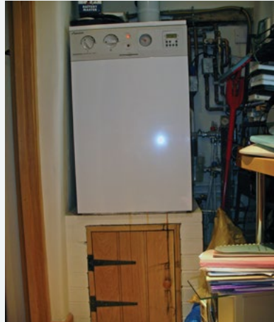
Figure 4 Boiler on plinth
