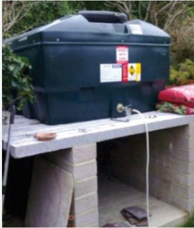
Figure 3 Fuel oil tank on raised plinth
