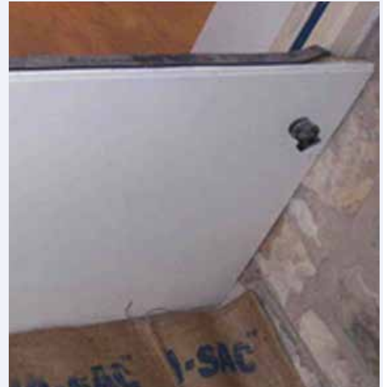
Figure 3 Door guard fitted to the internal door way
